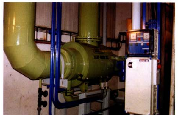
Filtration station of cooling water in a power station
