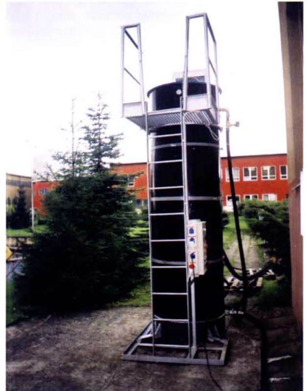
Continuously operating sand filter in paper mill, CR
