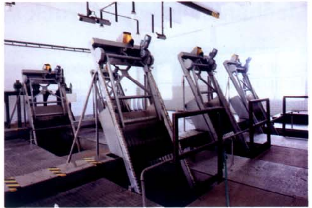
Truck screen in WWTP, Slovakia
