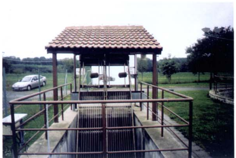
Truck screen in WWTP, CR
