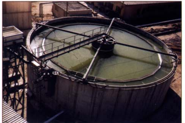
Thickening tank ZN 18/6
