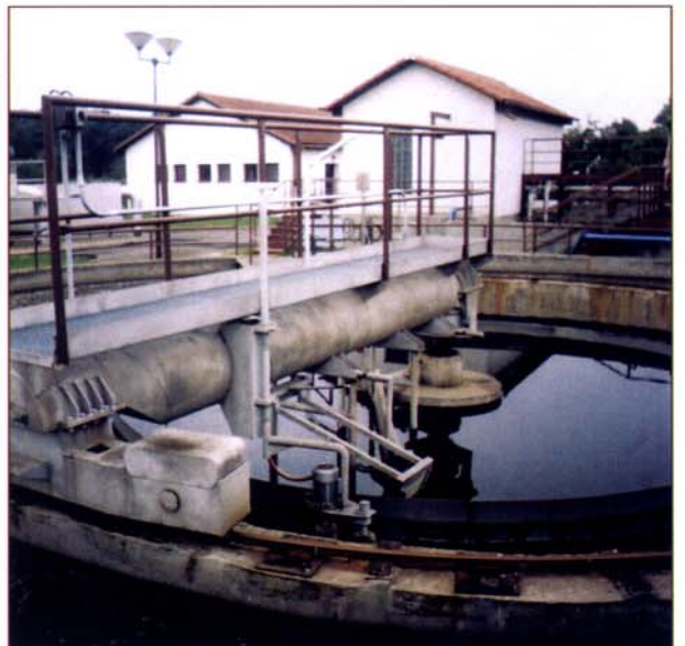
Secondary sedimentation tank in detail
