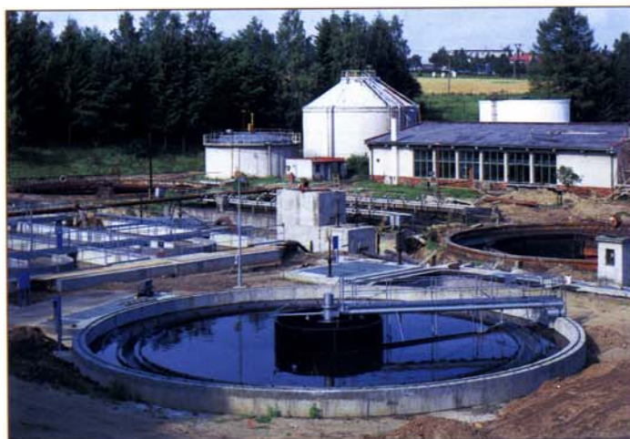
Secondary sedimentation tank at WWTP, CR
