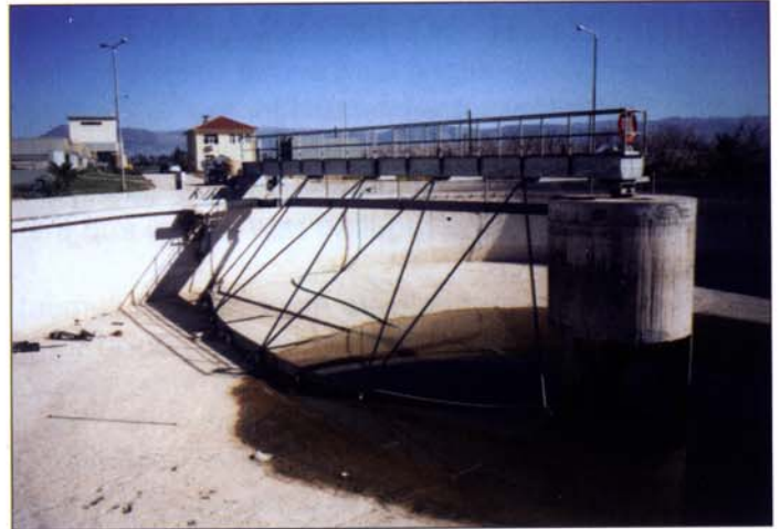
Secondary sedimentation tank at WWTP, Cyprus
