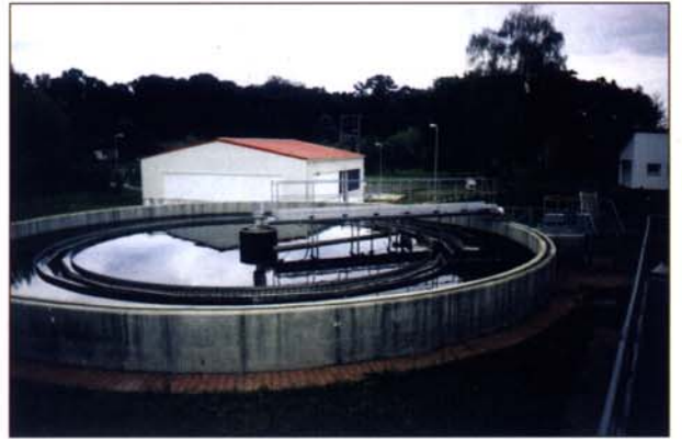
Secondary sedimentation tank DN-M
